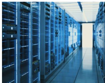
Freshwater > cooling data centers
